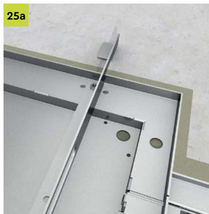
25a Check for complete relining by means of visual inspection of the holes of the cassette surface.
