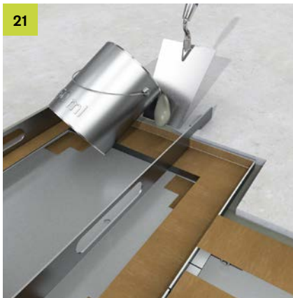
21 Backfilling with fast-hardening and low-shrinkage swelling grout or screed for highest loads (see note p. 11).
